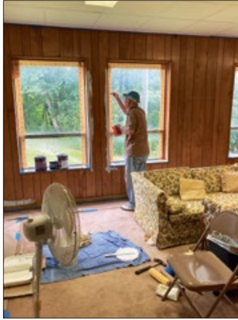
A St. John member helps renovate a dingy unused room into a bright new space for ministry.
