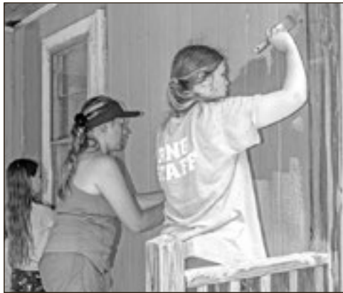
Grace UMMen joined forces with church youth to complete three days of community home repair projects.
