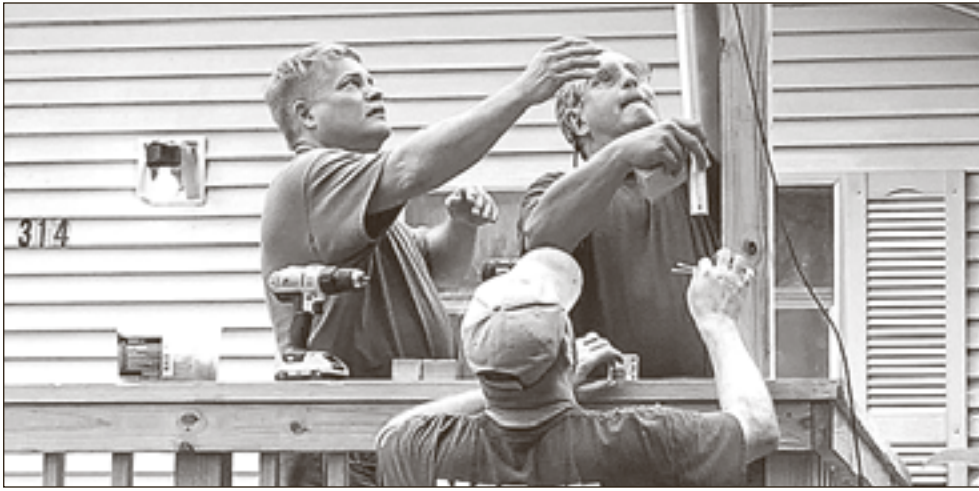
The 8- by 16-foot new porch has steps, railings and a pole for a TV antenna.
