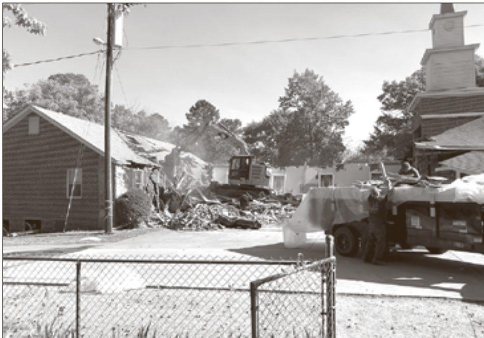
The former Lynnwood UMC property was demolished after structural issues were discovered. The "Eubanks Cross" was relocated to the new Grace-Lynnwood UMC property, and the cornerstone was relocated to the new site of The Bridge.
