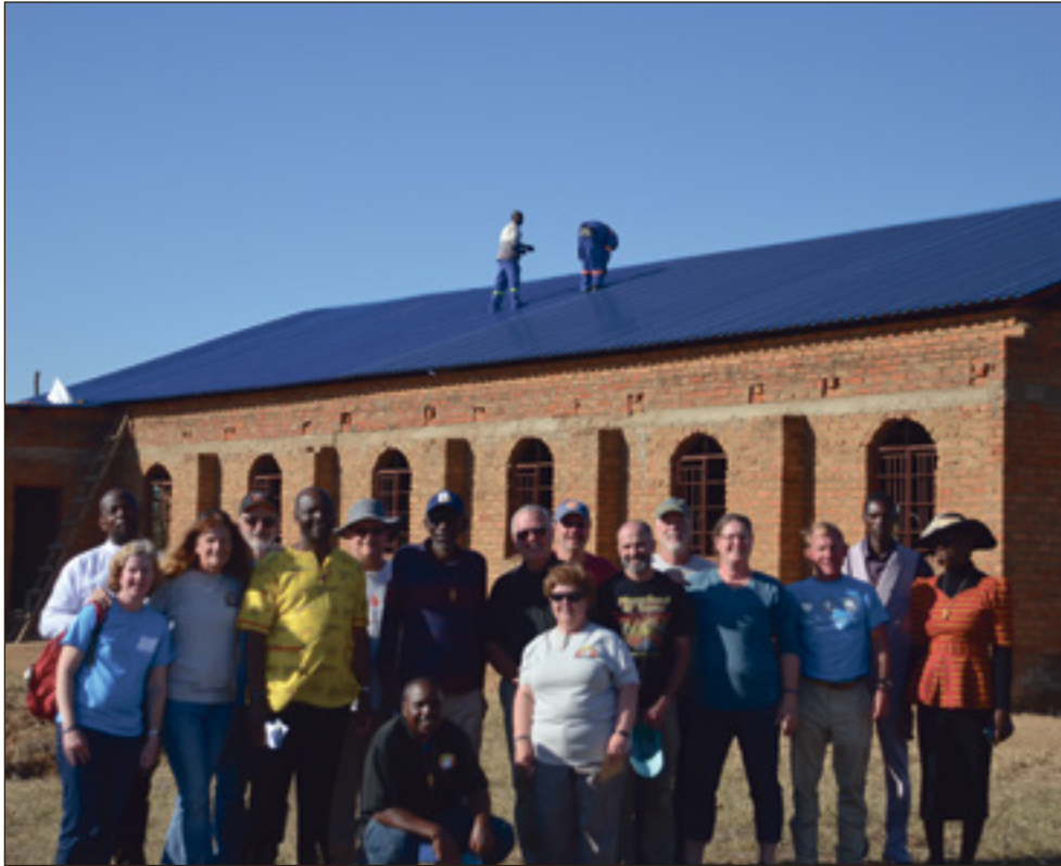
The team from Union UMC, Irmo, and leaders of the church gather in front of the completed roof.
