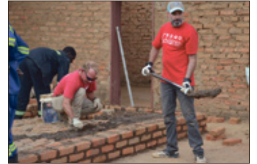
Chris Elvis (right) and Stuart Hope (left) spread concrete on the chancel area.
