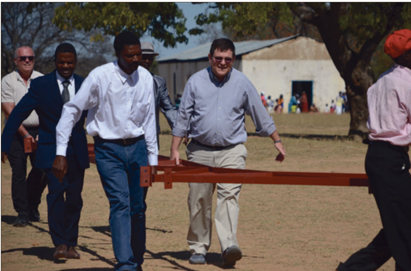
Chris Lindler (center) and Vic Caldwell (back) help the men of Chitenderano UMC carry a truss to the new church.
