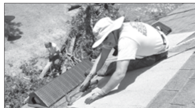
ERT member Felix Vazquez hammers on the roof as the Rev. Fred Buchanan chainsaws below.
