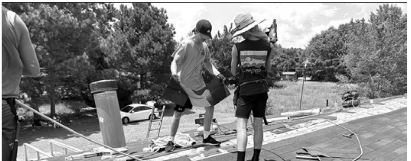
Youth volunteers at one of the Santee homesites didn't let the heat stop them from putting a new roof on a man's home during one of the hottest weeks of the year.
