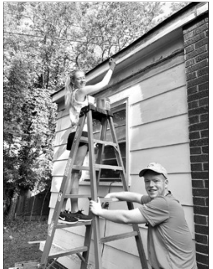
Safety first! A volunteer holds a ladder for another working on a roof at the Rock Hill camp.
