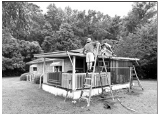
Volunteers at this homesite, part of the Santee Camp, repaired one roof and re-shingled another.
